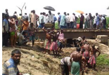
People are cutting the earth to widen the Rail & Dhaka-Khulna high way on self-labour
