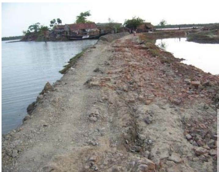
Photo: Damaged road in Koyra
